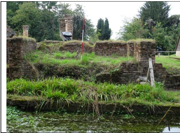
Middle of south wall (F-G) showing collapsed brickwork and temporary prop before work 2021
