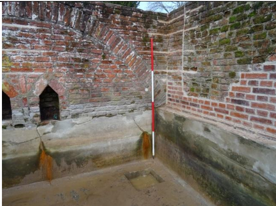
Sump in north east corner of cellar
